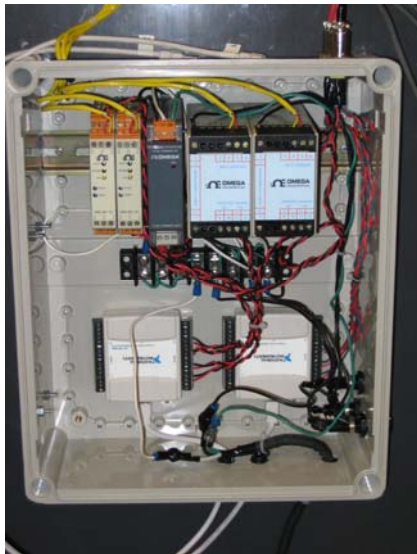
Figure 11. Data signal conditioning and acquisition box
