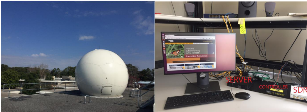
Figure 5: S-band station at CCRF. First photo shows a 3m dish antenna system covered by a radome. Second photo shows the workstation next to the antenna system, with SDR and antenna controller connected to the server, through USB 3.0 connector and Ethernet cable respectively. SDR is connected to a RF cable, which goes to the RF hardware system within the radome.
